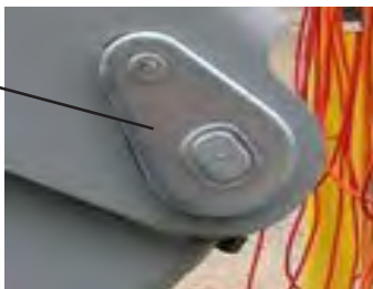
No rust. Pin has not rotated. Area is clean of dust/metal shavings
